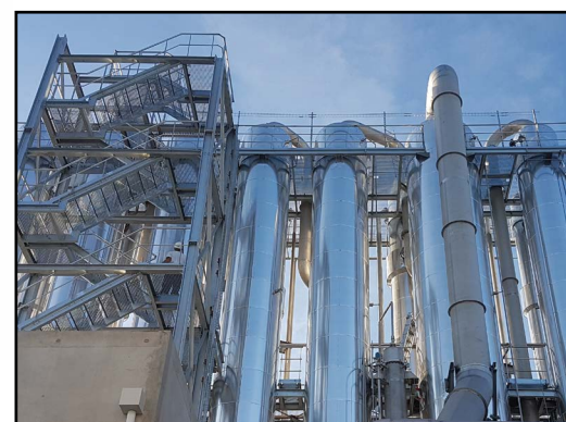
Multiple effect evaporation plant
